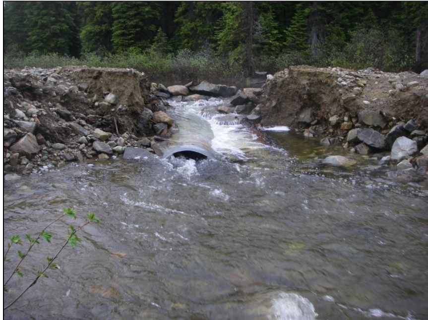
PHOTO I6 – T-Creek hydrology station (TSFUS), upstream road and culvert washed up
