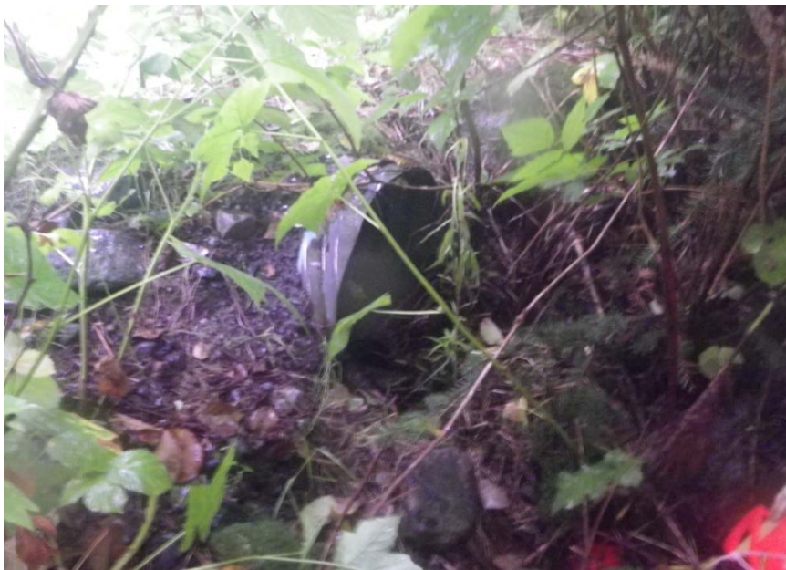
Photograph 20: WC 17 looking north upstream at 600mm culvert crossing underneath the main road. July 14 th , 2011
