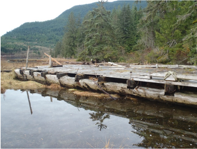
Photograph 10: Old wharf debris.
