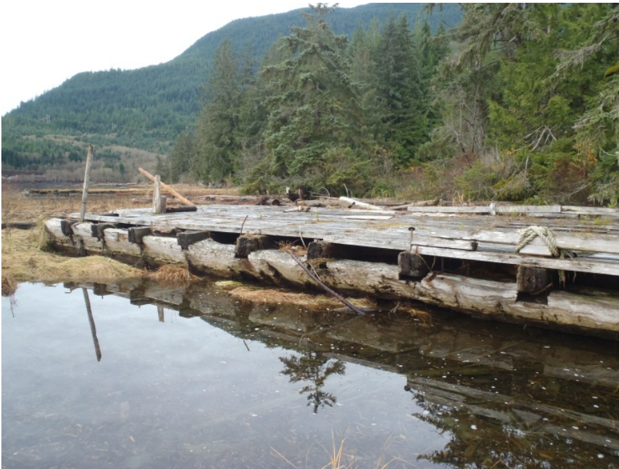
Photograph 13: View of abandoned log-based float.
