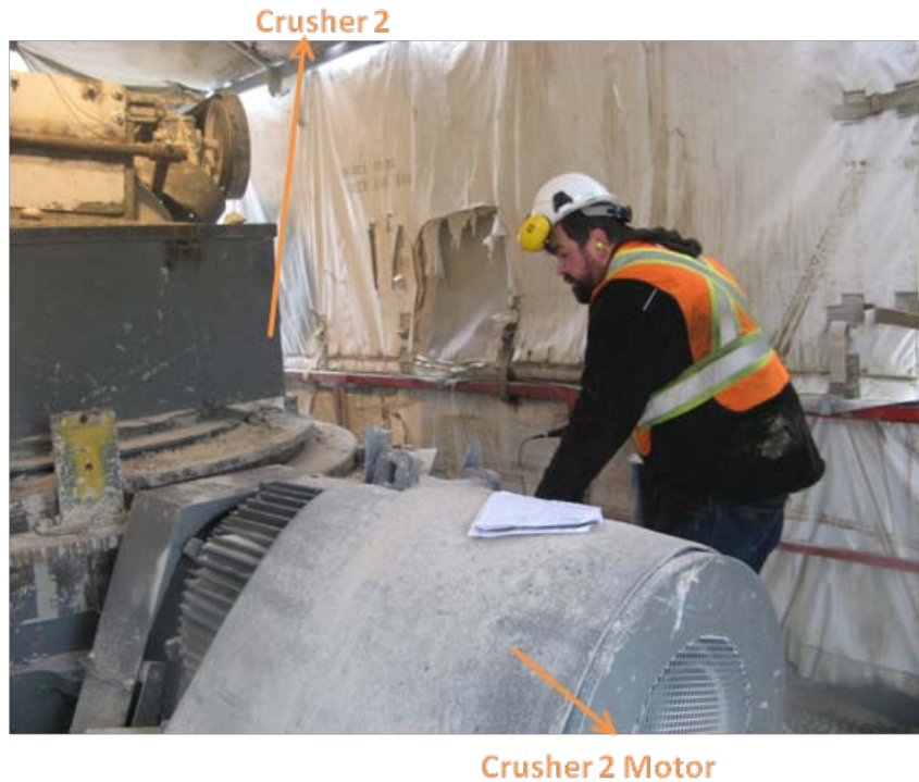
Photo 4: Inside the Canvas Shed Housing Crusher 2 and its Motor
