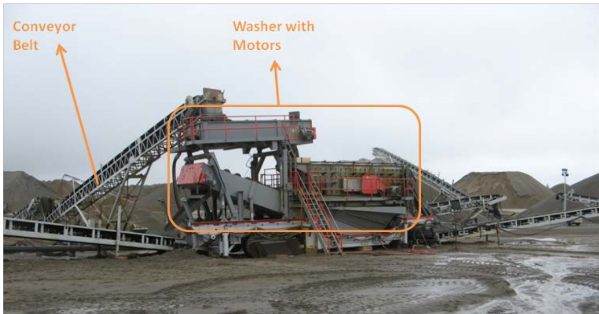
Photo 12: Washer Unit in the Wash Plant
