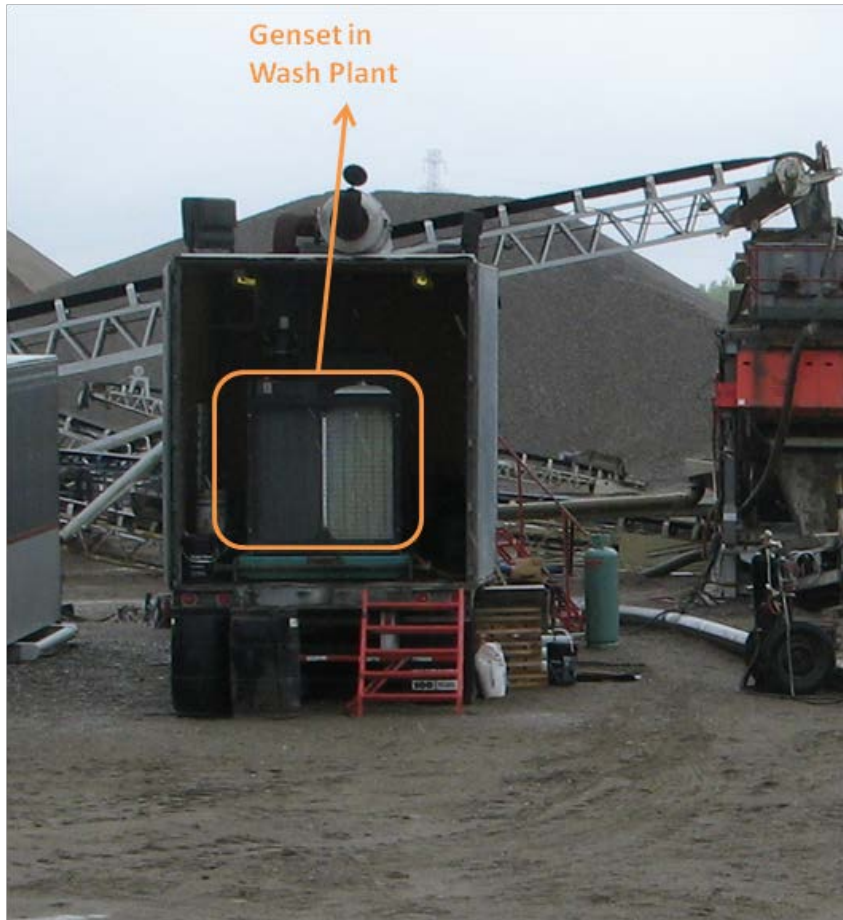
Photo 11: Genset 3 in the Wash Plant
